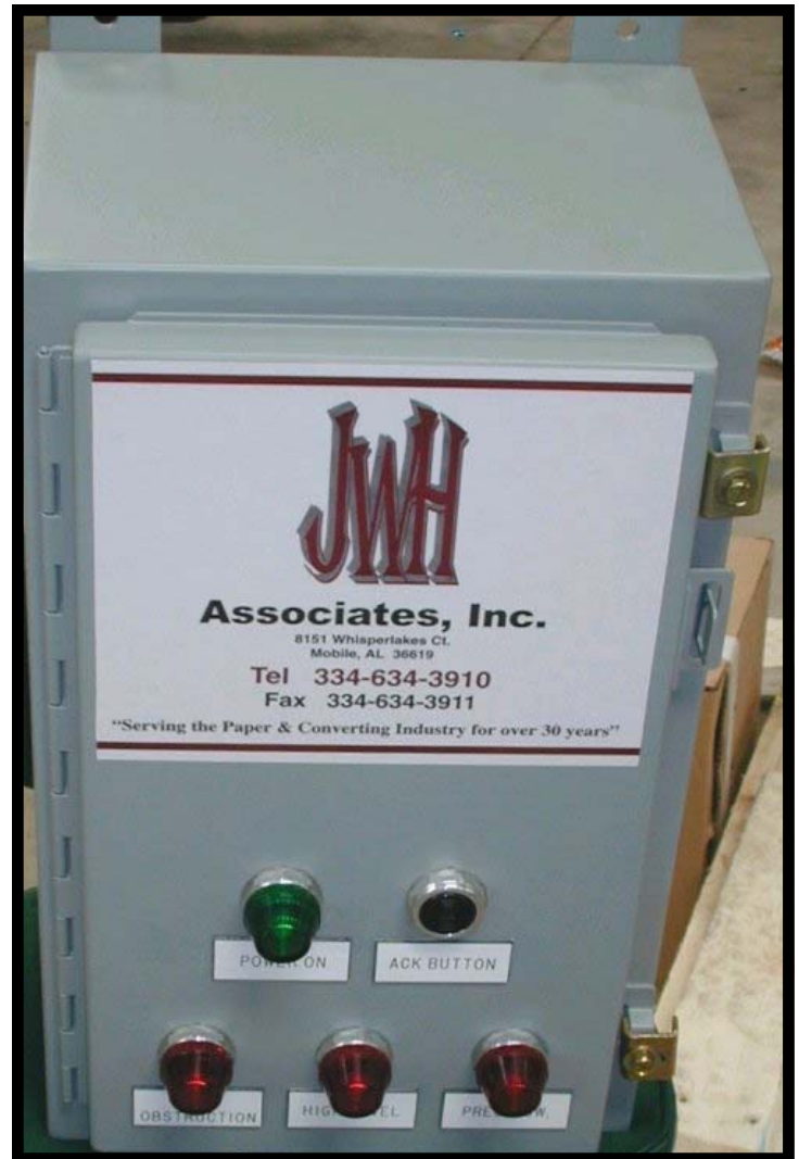
PEWS Control Panel
